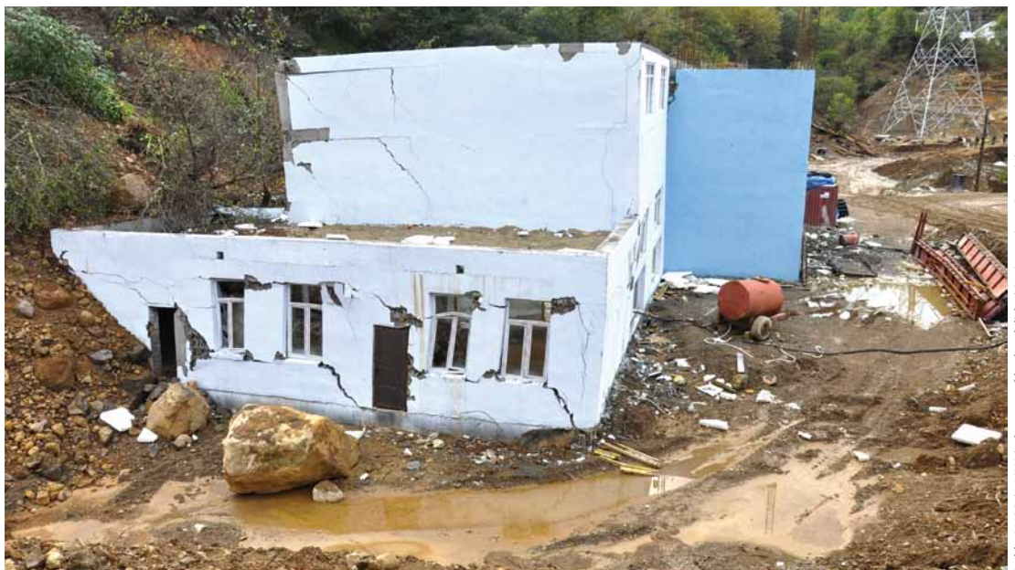
Bakhvi HPP (6 MWt) destroyed by landslide (Guria region, Georgia). Author: Green Alternative.
